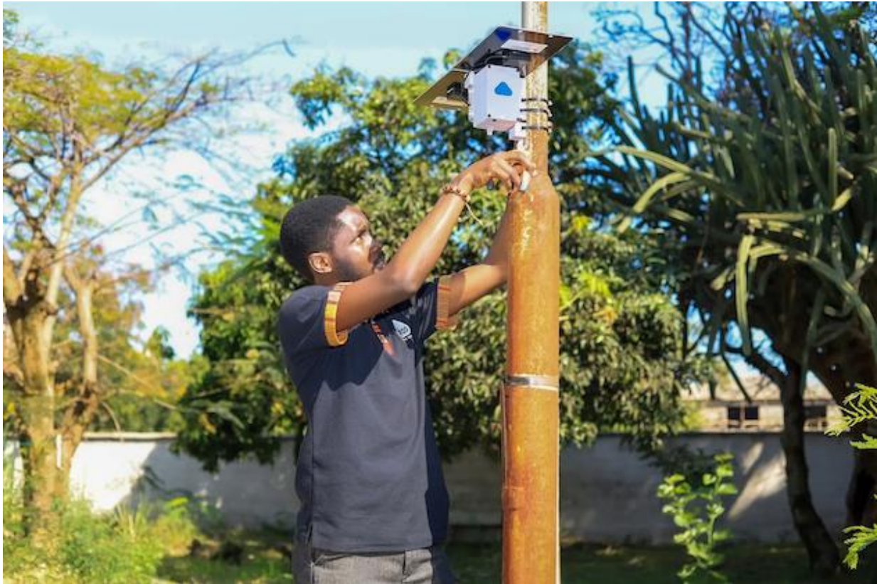
A technician installs a low-cost air quality monitor sensor in Nairobi, Kenya. Air quality monitors are helping Nairobi collect data on air pollution. Credit: Jackson Okata/IPS
